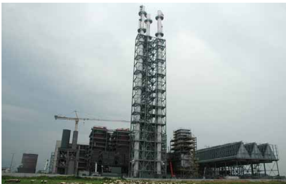
Fig. 2 Incinerator of Acerra, Naples
